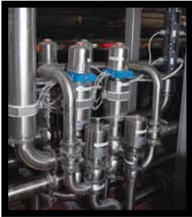
The new mix-proof valves, larger pumps, variable drives with flow meters and flow based sampling have increased throughput in receiving to five-million pounds per day.
