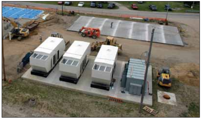
The generator pad is complete and the new back-up generators are being installed. With the addition of new electrical hook-ups and controls, the generators will have the capacity to run the existing plant in the event of a power outage. Three generators are scheduled to be online by the end of 2009 and generate two megawatts of electricity per unit, totaling six megawatts of capacity.
